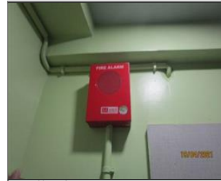
Photo of fire safety equipment fire alarm.JPG
