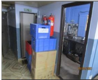
Photo of non-conformity fire extinguishers were found blocked.JPG
