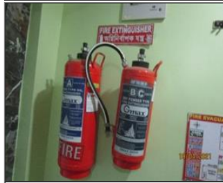
Photo of fire safety equipment fire extinguisher.JPG
