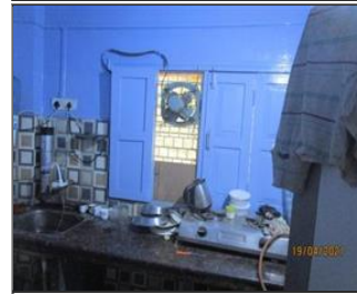
Photo of non-conformity exhaust fan was not fenced.JPG
