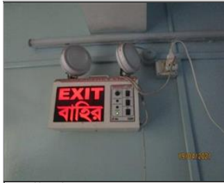
Photo of fire safety equipment emergency light.JPG
