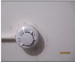
Photo of fire safety equipment smoke detector.JPG
