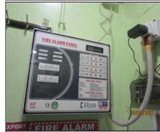
Photo of fire safety equipment fire panel.JPG
